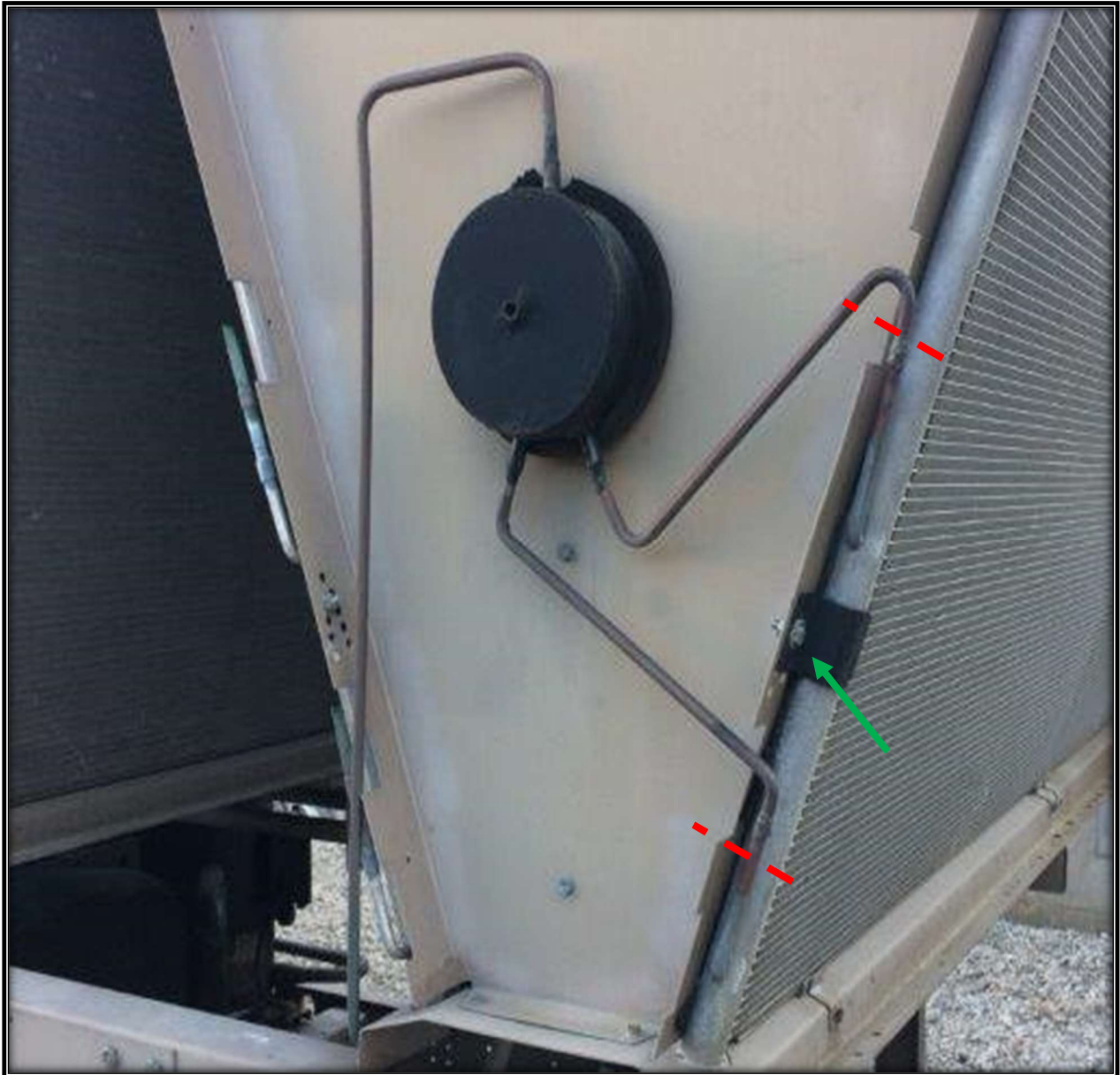
Figure 3. Back of Chiller: Cut existing receiver lines as shown in Red. Unbolt the coil at 4X locations as shown in Green.
