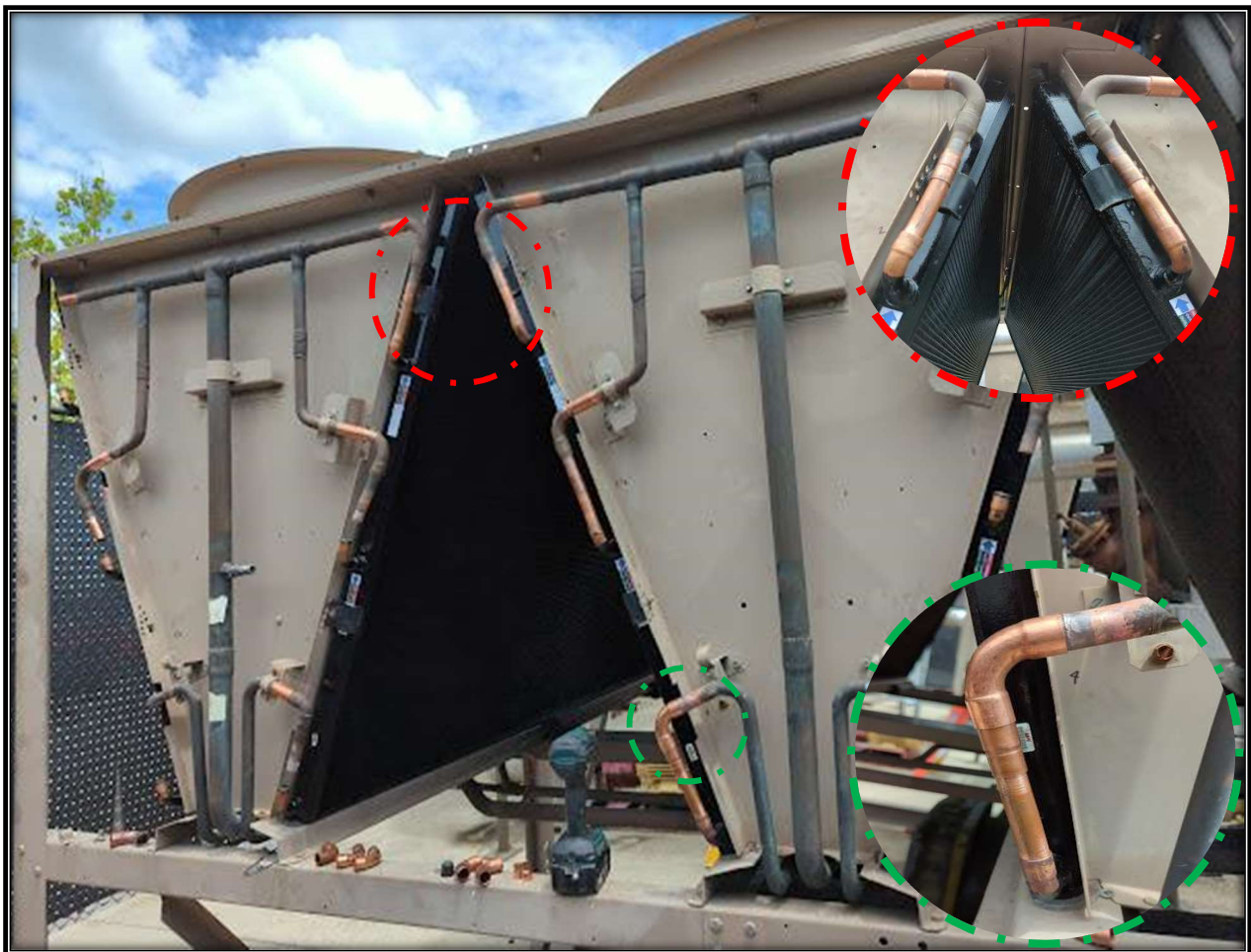
Figure 4. Front of Chiller: Solder Copper Connections as Shown.
