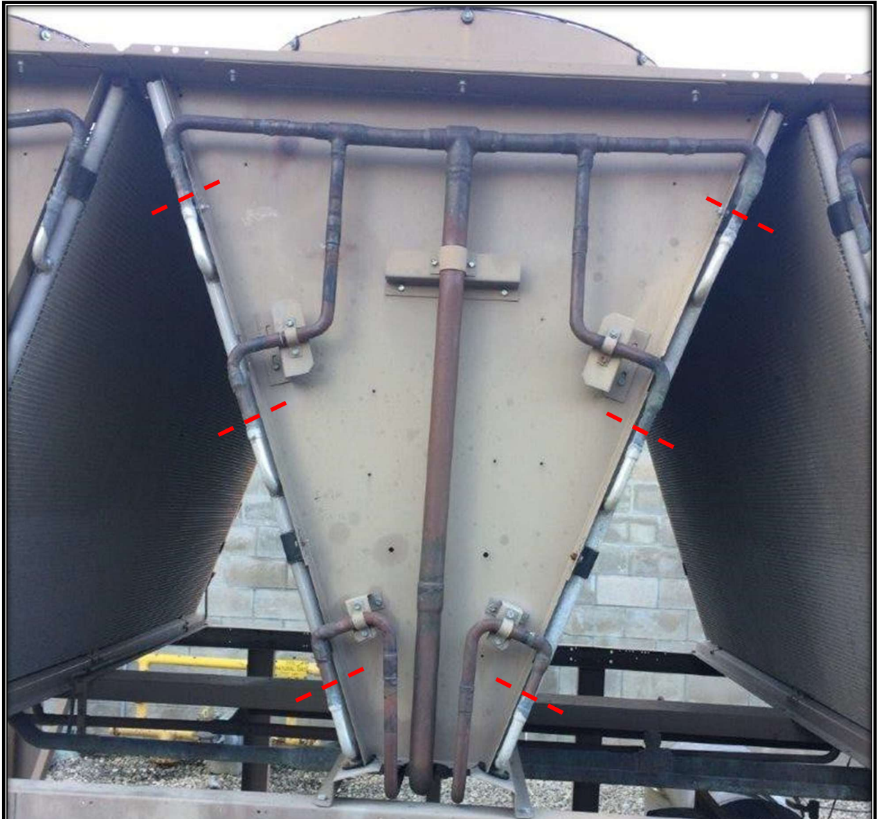
Figure 2. Front of Chiller: Cut Existing Discharge and Liquid Lines as Shown in Red
