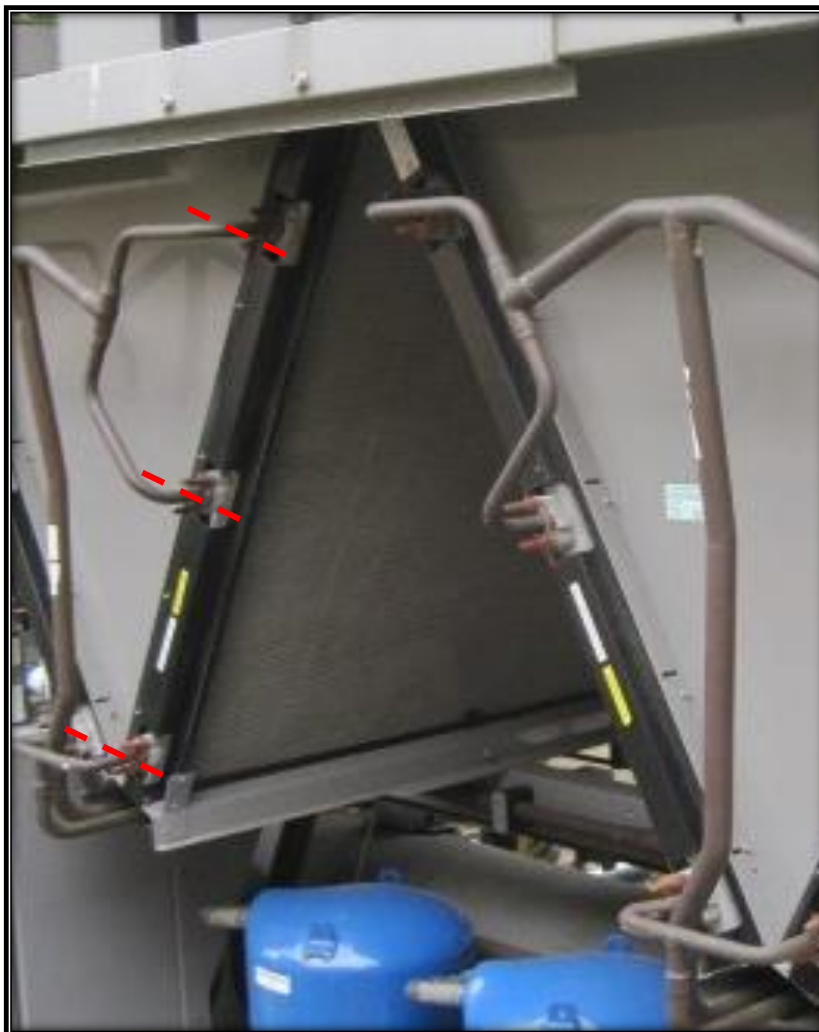
Figure 5. Cut Discharge and Liquid Lines as Shown in Red.
