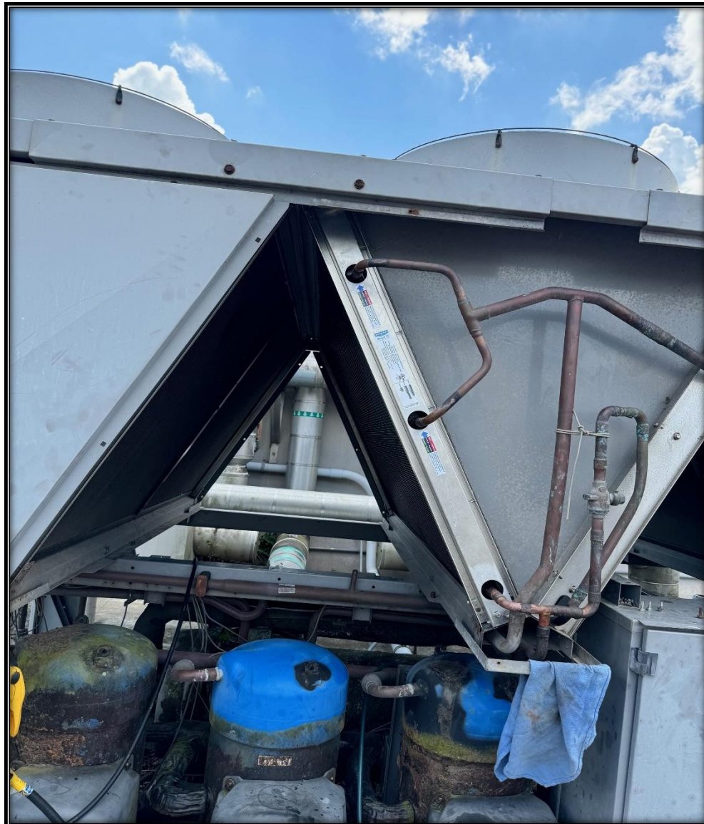
Figure 8. Front of Chiller: Solder Connections as Shown.
