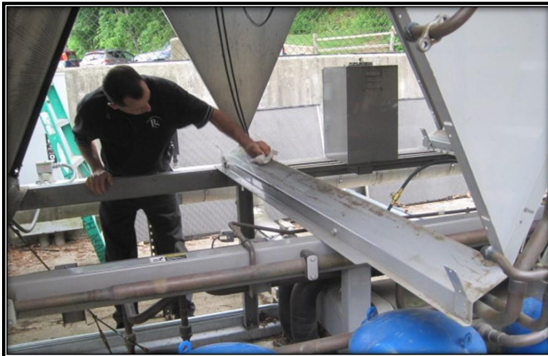
Figure 4. Clean Upper and Lower Coil Supports
